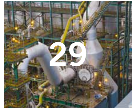
Blast furnace gas cleaning and recovery systems
