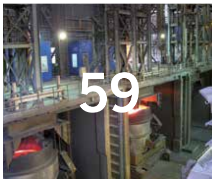
Hot metal desulphurization systems
