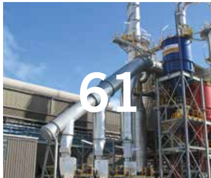
Fume treatment centers for aluminum smelters
