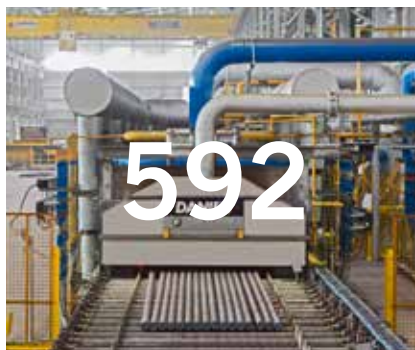
Heat treatment furnaces
