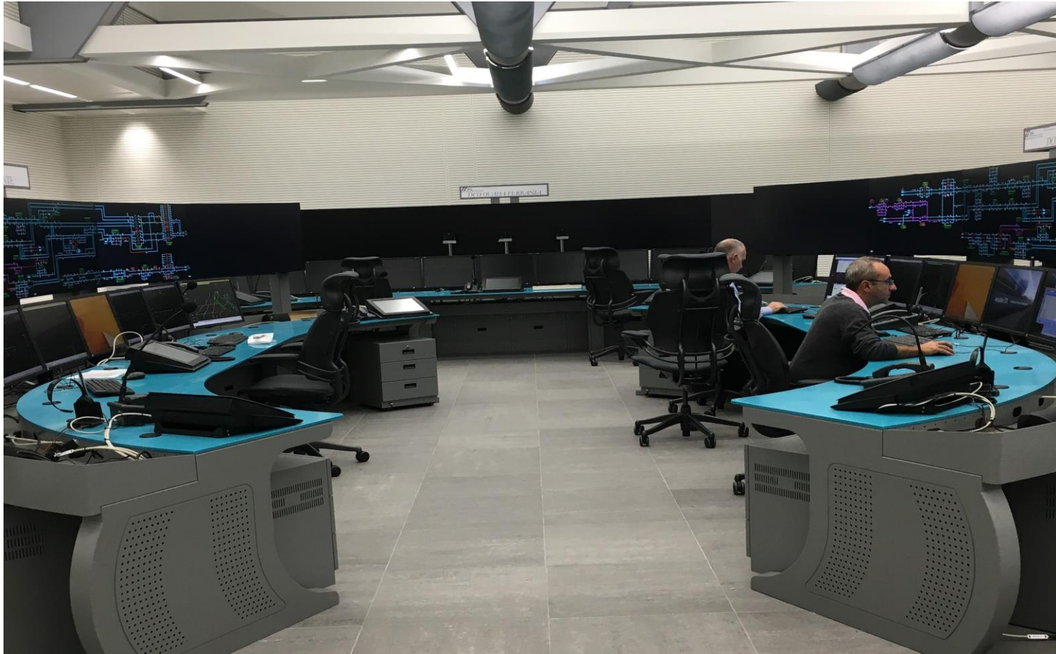
The Rail Traffic Operating Centre of the Genoa, Liguria and Basso Piemonte railway junction
