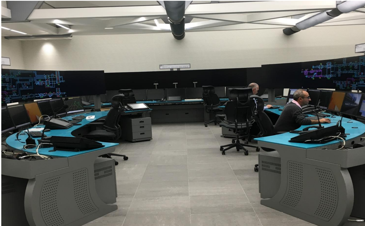
The Rail Traffic Operating Centre of the Genoa, Liguria and Basso Piemonte railway junction
