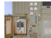
Power Conversion, & Distribution
