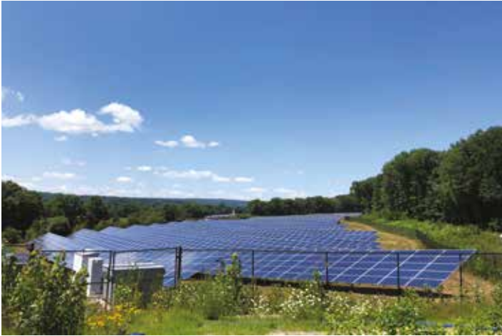
Massachusetts photovoltaic plant
