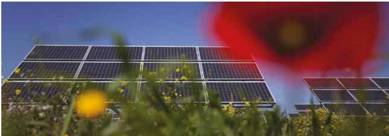
Notarpanaro (Solar Mesagne – Brindisi) photovoltaic plant
