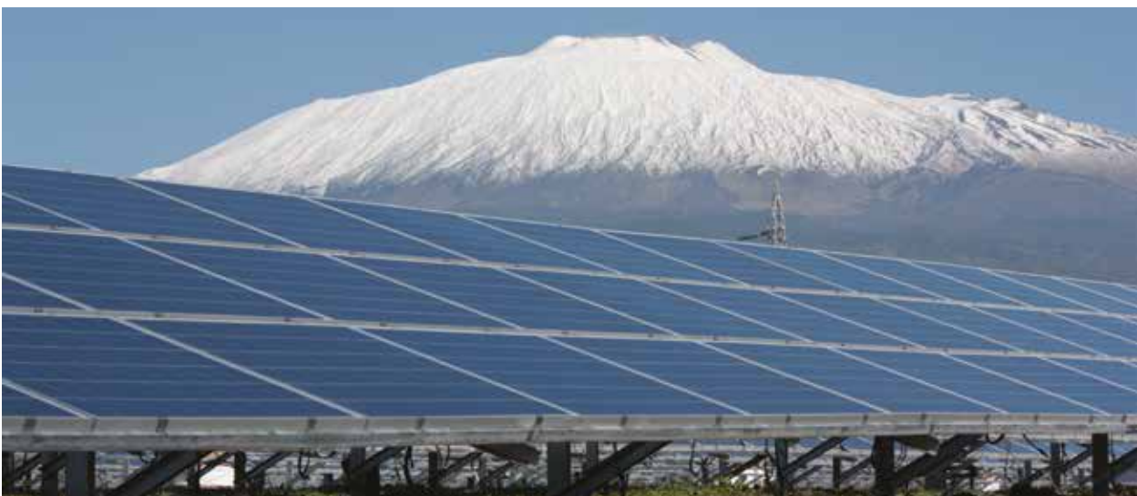
Cardonita – Centuripe (Enna) photovoltaic plant
