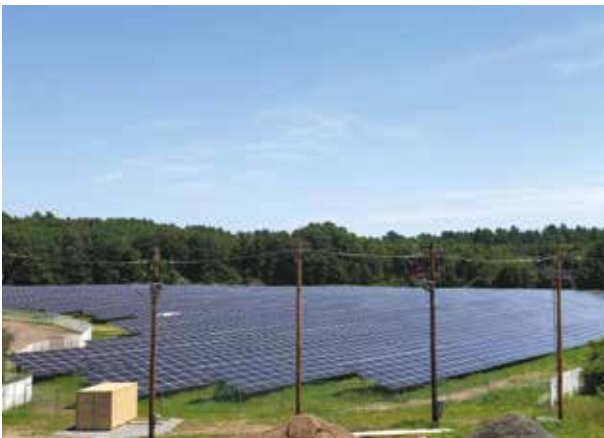
Middleton (Massachusetts) photovoltaic plant
