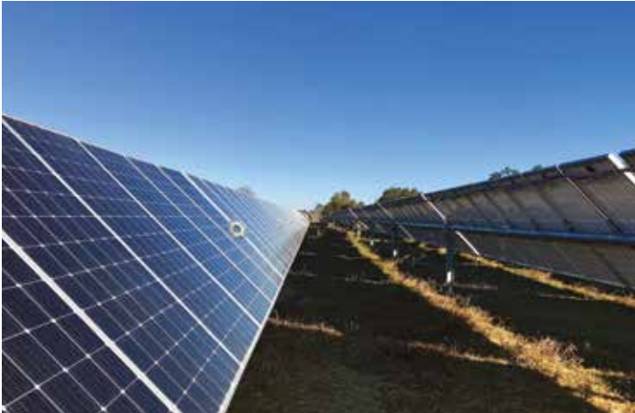
IS42 (North Carolina – USA) photovoltaic plant
