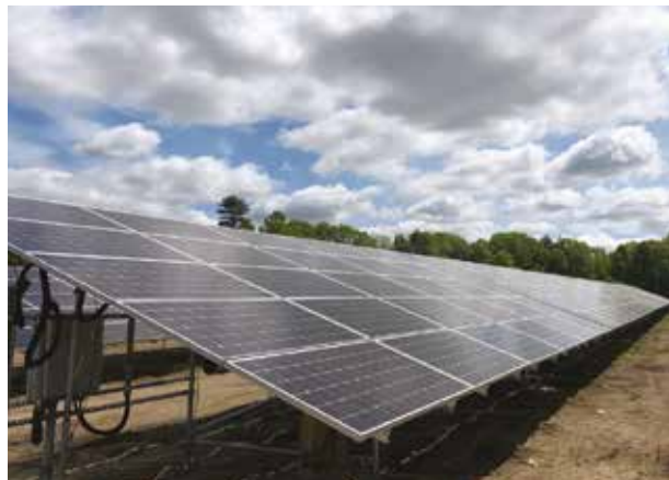
Middleton (Massachusetts) photovoltaic plant
