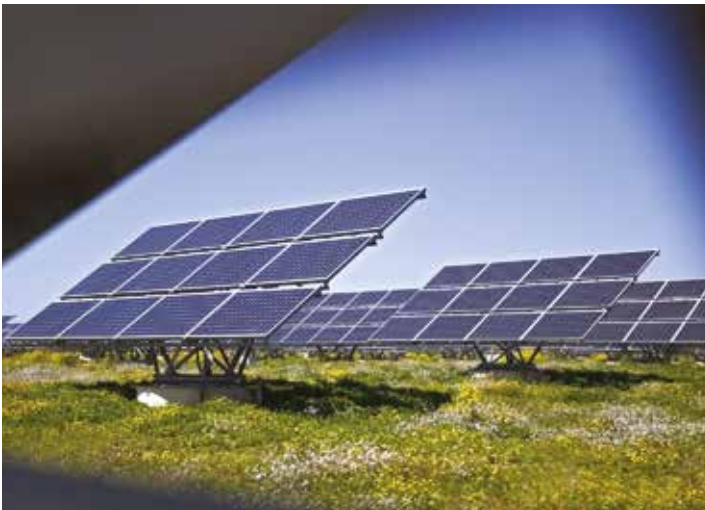
La Calace (Solar Mesagne – Brindisi) photovoltaic plant
