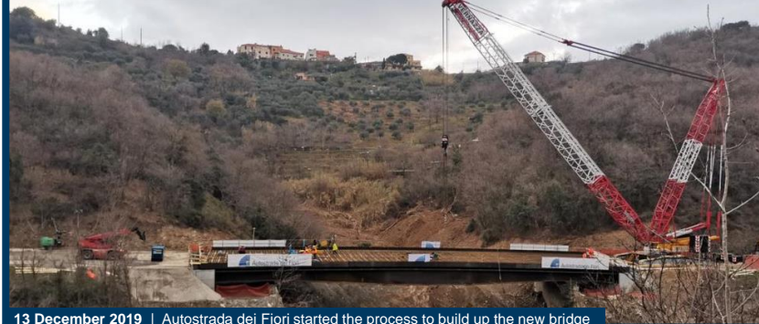
13 December 2019 | Autostrada dei Fiori started the process to build up the new bridge
