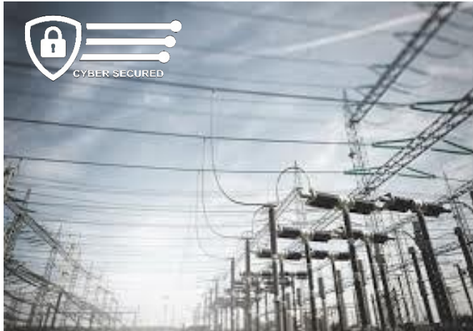
Awarded tenders for protection and control solutions to properly secure the electrical grid
