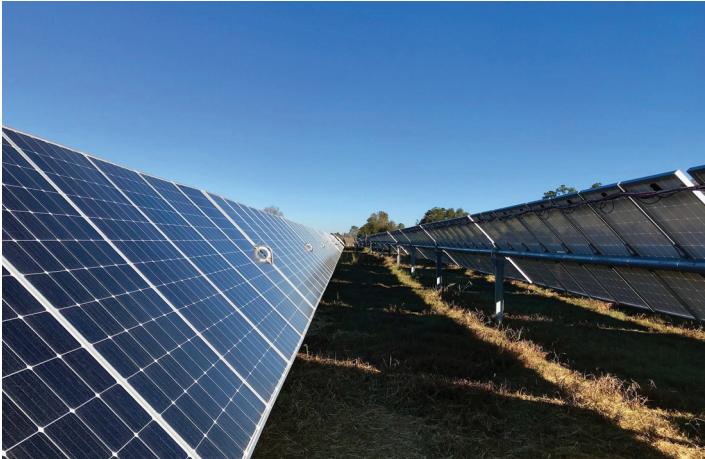
IS42 (North Carolina) photovoltaic plant
