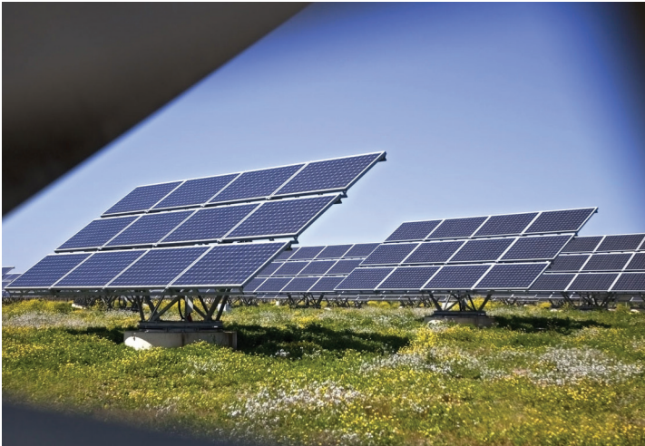
La Calce (Solar Mesagne-Brindisi) photovoltaic plant
