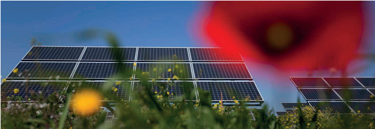
Notarpanaro (Solar Mesagne-Brindisi) photovoltaic plant
