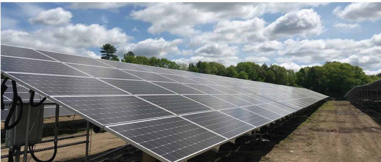
Middleton (Massachusetts) photovoltaic plant
