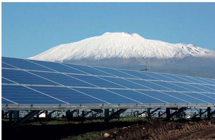
Cardonita-Centuripe (Enna) photovoltaic plant
