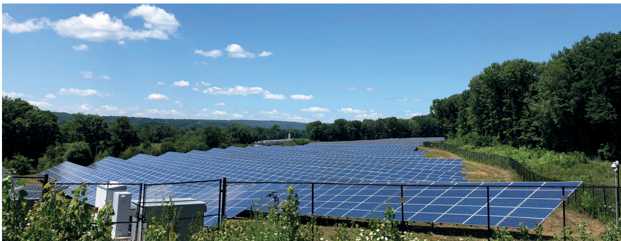
Leominster (USA) photovoltaic plant
