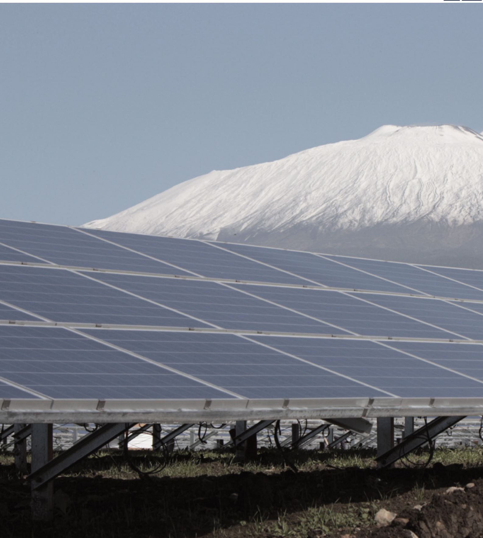
Cardonita - Centuripe (Enna) photovoltaic plant.
