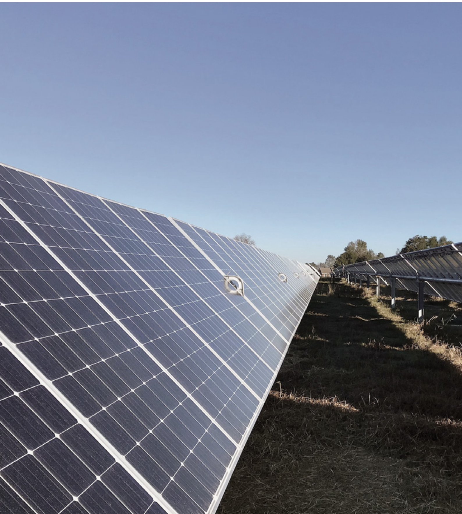
IS42 (North Carolina) photovoltaic plant.
