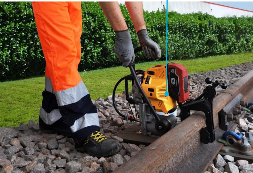
Sleeper drilling machine
