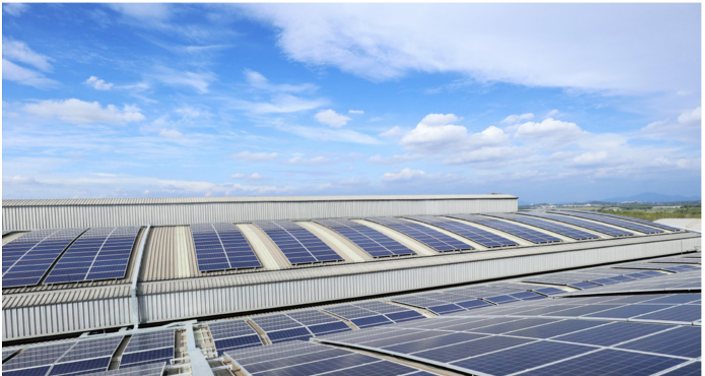
Photovoltaic installations at the Empoli technology centre
