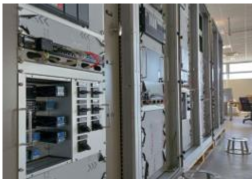
Significant progress in the development of Substation Automation solutions
