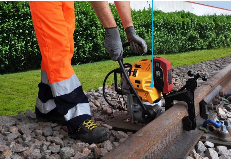
Sleeper drilling machine
