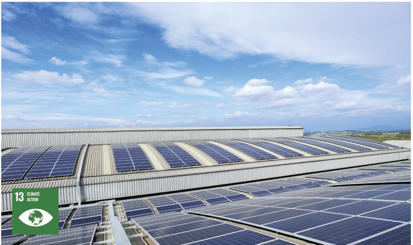
Photovoltaic installations at the Empoli technology centre
