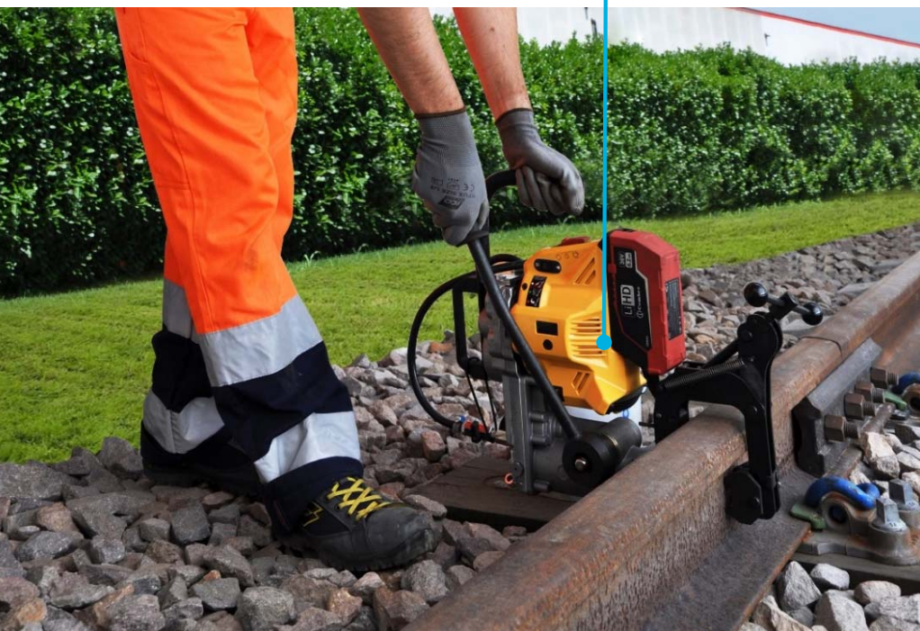
Sleeper drilling machine
